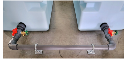
Tank Connection Manifold
