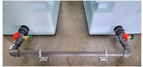
Tank Connection Manifold
