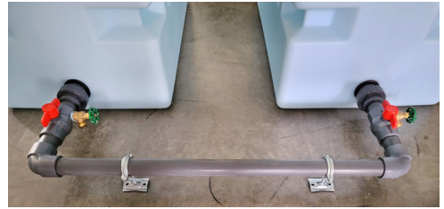
Tank Connection Manifold
