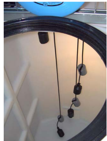
Inside of 425-gallon Well Manager tank with Stop Loss installed. The two floats on the right operate the Stop Loss solenoid.
