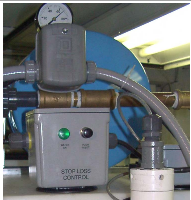
Stop Loss Control Mounted on a 425-Gallon Tank
