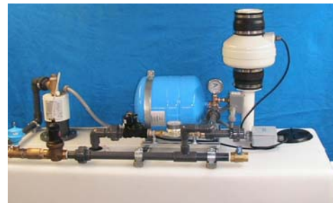
System with a Spray Boom and exhaust fan wired to run during fill cycles or constantly
